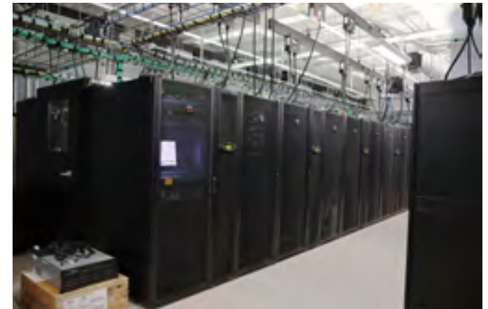
Public Safety Complex servers
