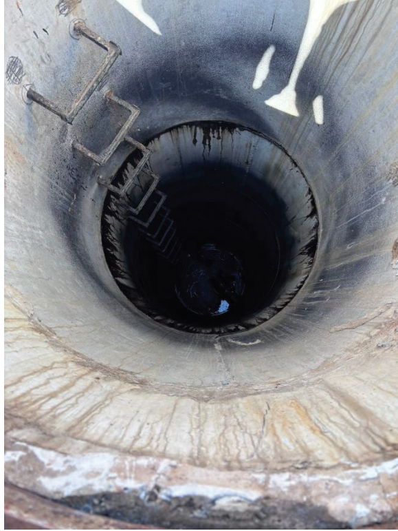
View of Vault for Float Valve
